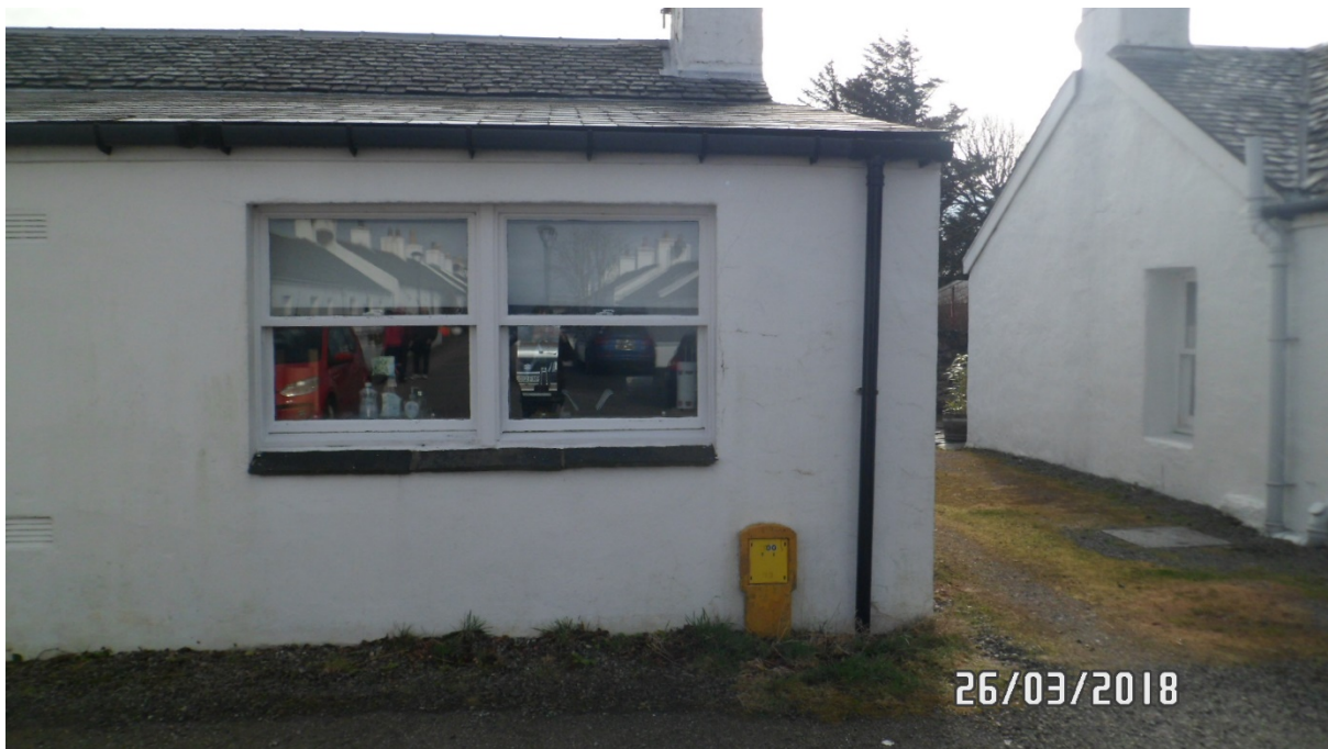
Close up of double white painted timber sliding sash and case window to rear elevation
