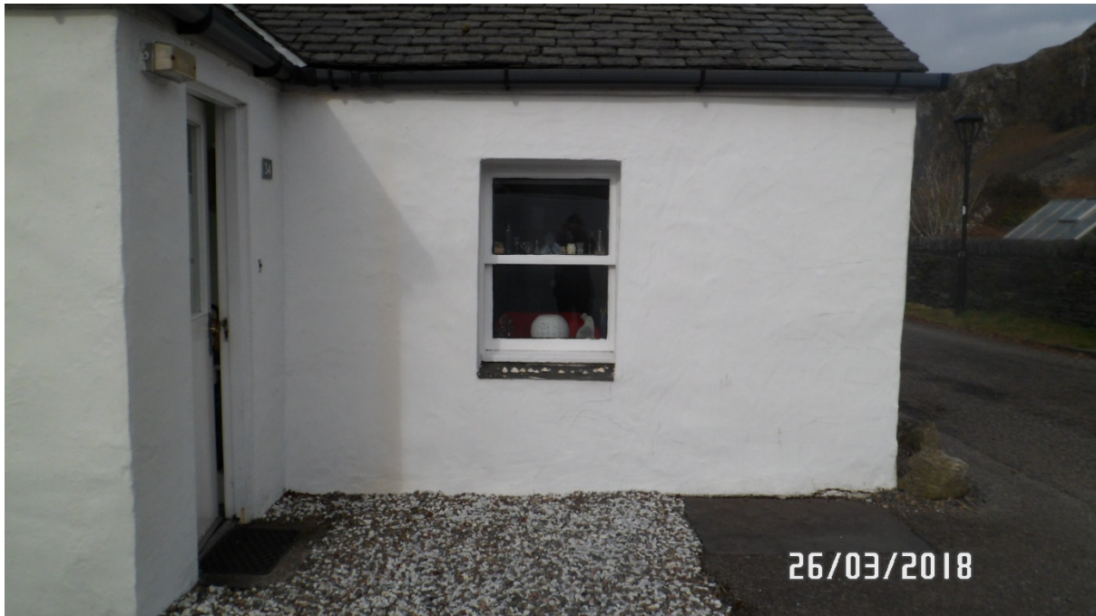
Close up of white timber sliding sash and case unit to front elevation
