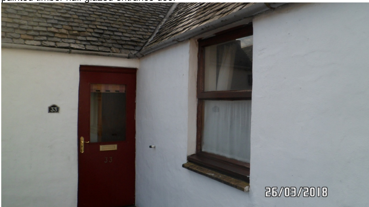
Close up of front elevation showing brown painted timber entrance door and brown painted timber top hung window
