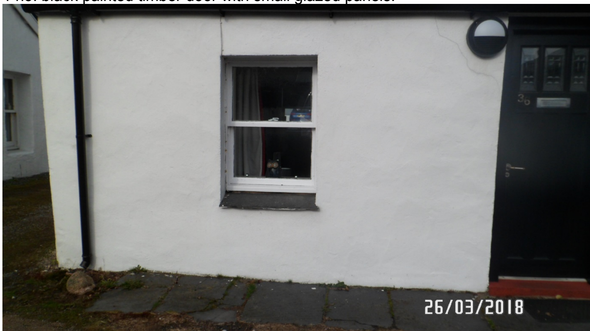
Close up of white painted timber sliding sash and case window to front elevation
