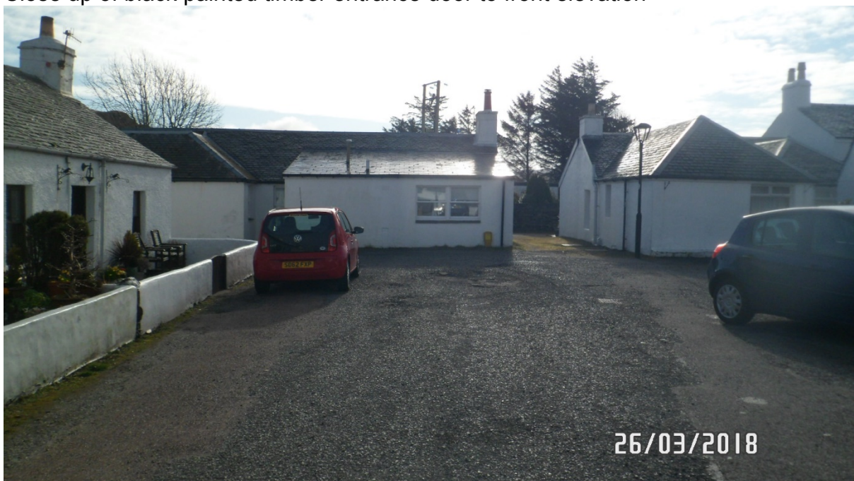
Rear elevation showing 2 no. white painted timber sliding sash and case windows, one double unit and one single unit
