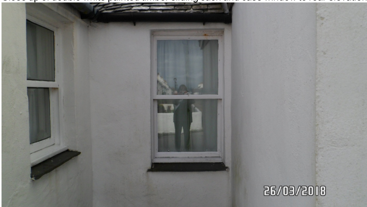
Close up of single white painted timber sliding sash and case window to rear elevation
