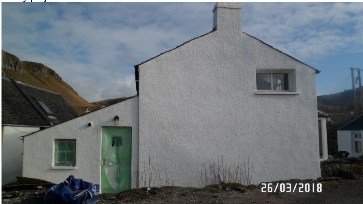
Side elevation showing 1 no. white painted timber unit at first floor the method of opening of which is not clear with 1 no. white painted timber door with glazing panel and 1 no. four pane white timber window to the side elevation of the single storey rear projection the method of opening of which is not clear.
